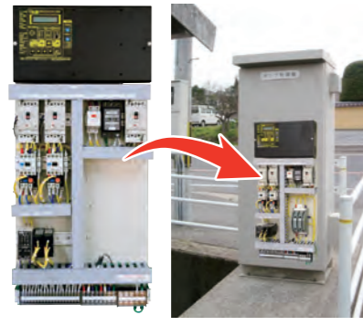
exchange unit of manhole pump control panel
