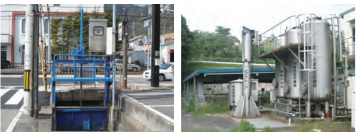
gate control system
