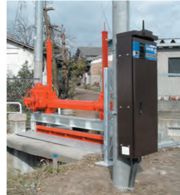
the gate management control system
